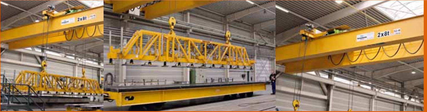
Double-girder bridge crane with load lifting device at the production halls of BUTTING
