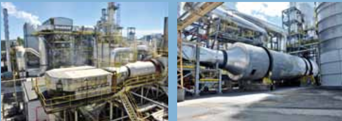
Energy plant (left) and particle dryer (right), Masisa Cabrero
