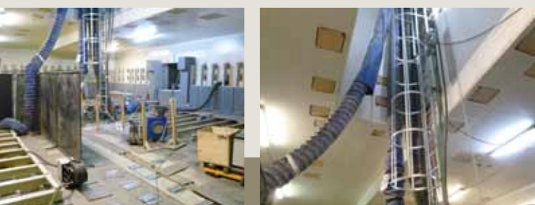
Venting hose for dust formation and vapors; ceiling opening of the venting hose: coevally entry for the cast elements, the lift truck etc.
