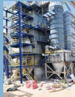
Energy plant (left) and fibre dryer (right), Panel Plus, Thailand
