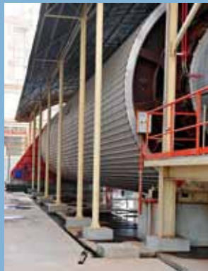
Energy plant (left) and particle dryer (right), Metro Thailand
