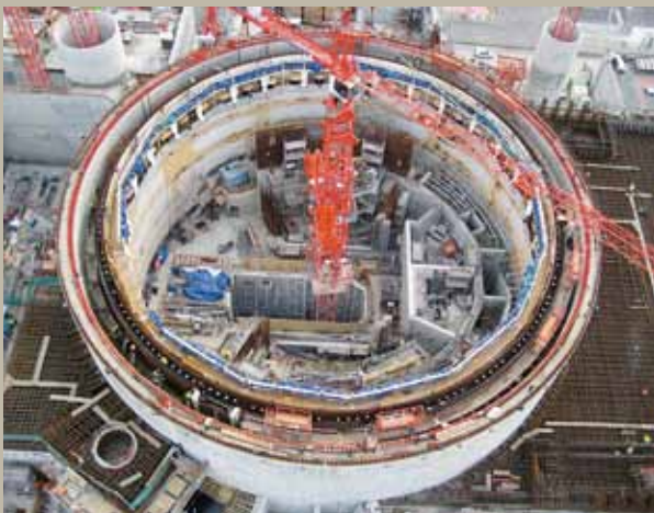
Reactor building under construction – deep inside, assembly of the core catcher cooling structure
