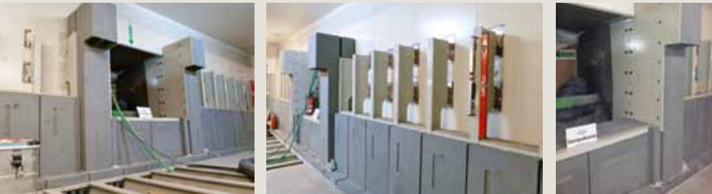
Mounted transition: inlet section between pressure vessel bottom side and core catcher for the conveyance of molten material
