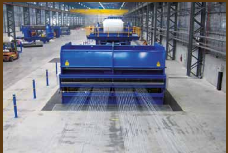
From the creel to the infeed area of the cable tensiing device
