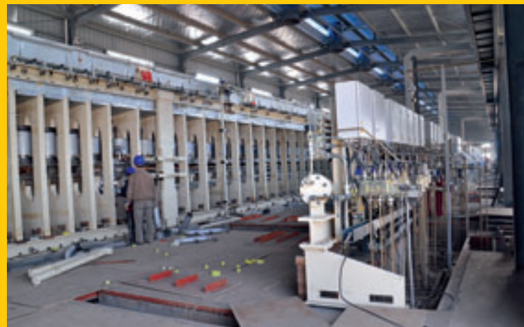
Hydraulics support next to the press
