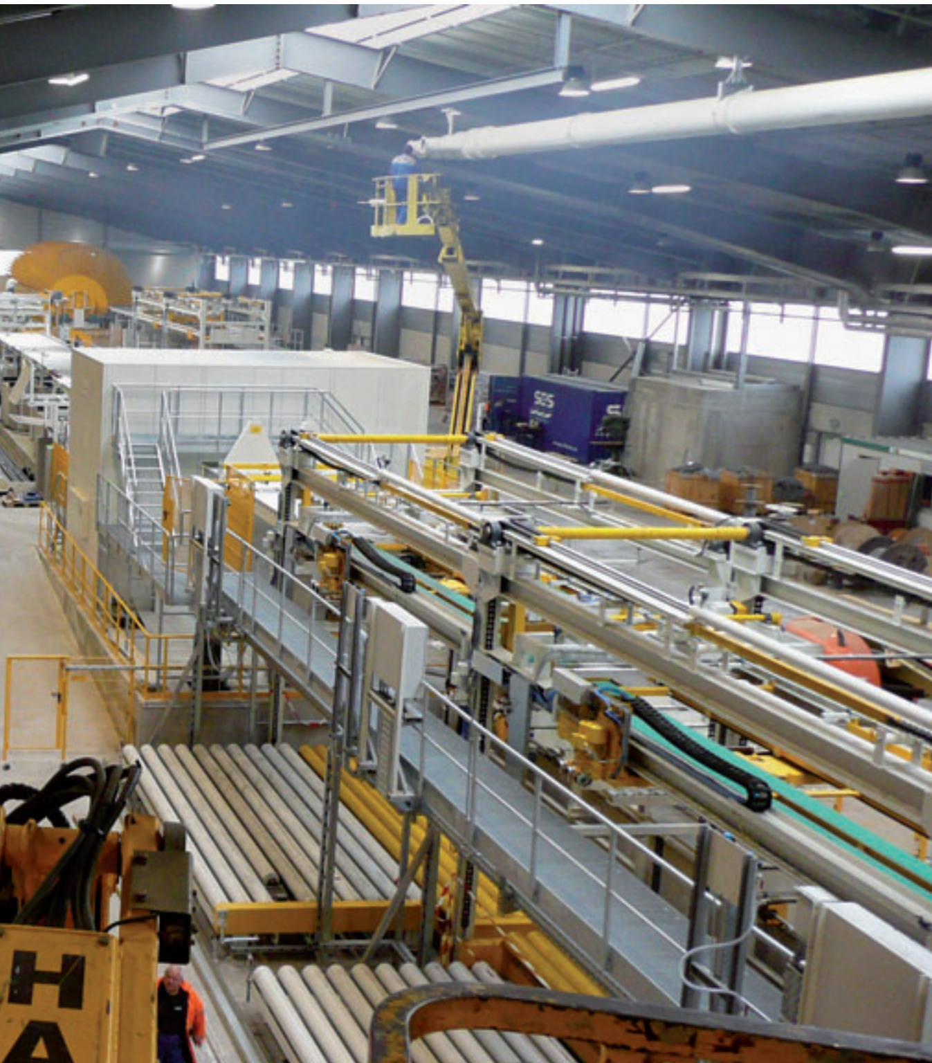
Finishing line with star cooler in the background
