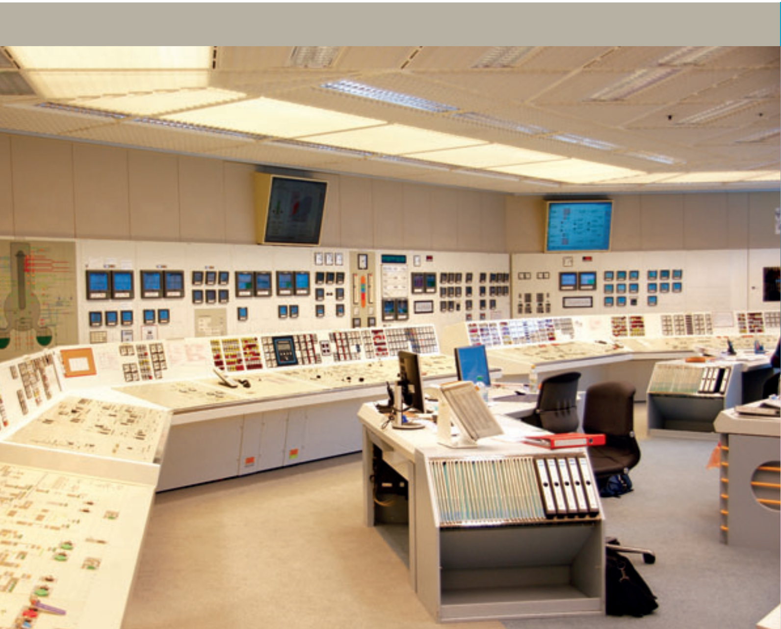
Main control room
