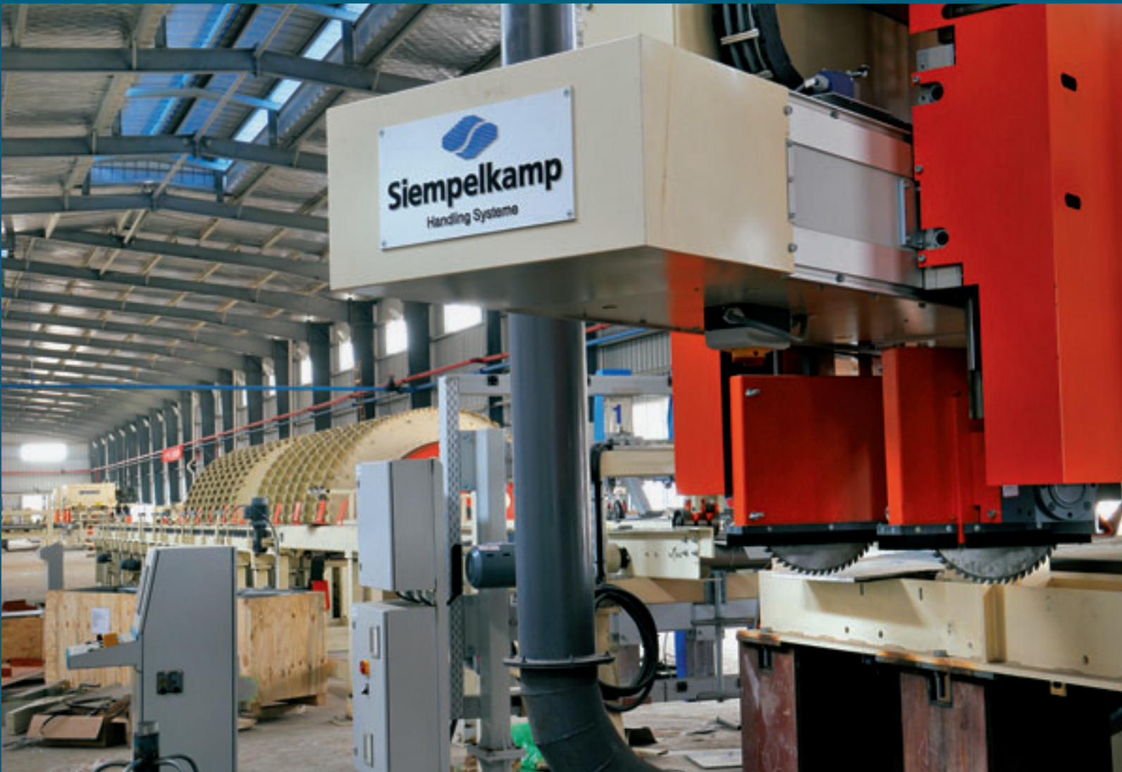
Double diagonal saw at the press outfeed area
