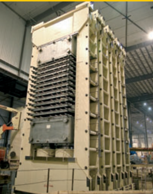
Largest multi-daylight press (12 x 34 ft) for Canfor LP, Canada
